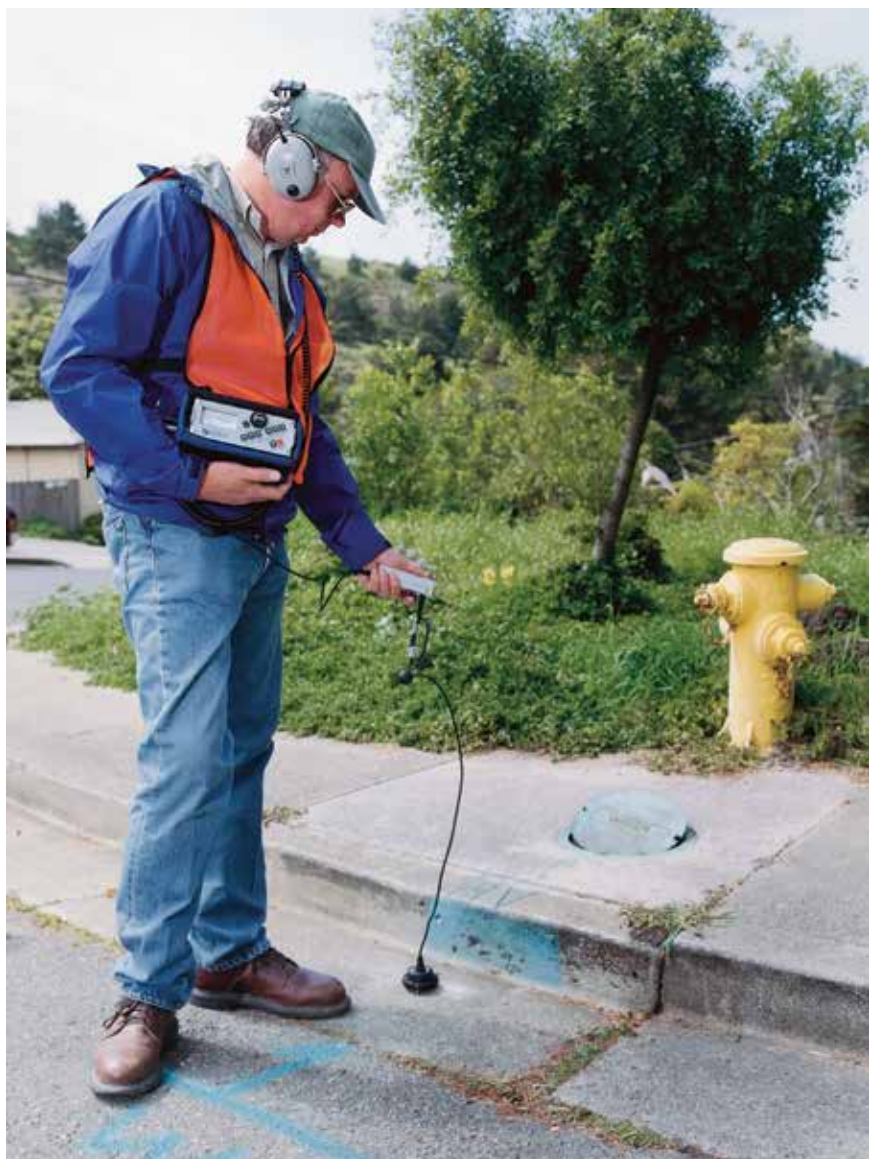
Figure 4-9 Leak Pinpointing Over a Hydrant Line
